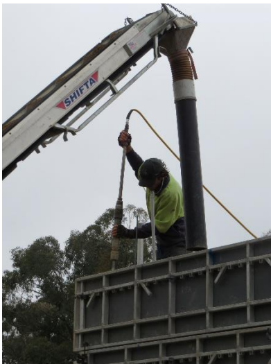
The rammed earth wall is immediately complete. The formwork can be removed shortly after the ramming is complete. There is no need to wait for it to become hard as you would with concrete. The finished wall is treated with to remove surface impurities and then sealed to control dust and moisture.
